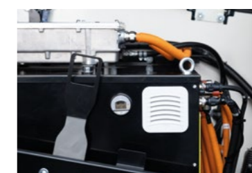
Battery compartment with monitoring system.
